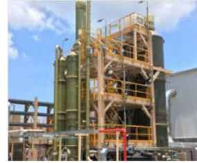
Wet Chemical Scrubber
