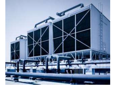
Heating & Cooling Systems
