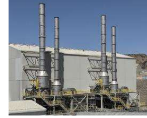
Particulate Scrubber / Cyclones
