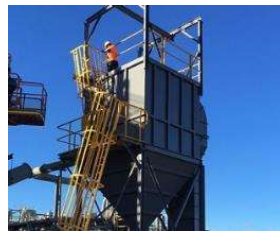
Fabric Filter (Baghouse)
