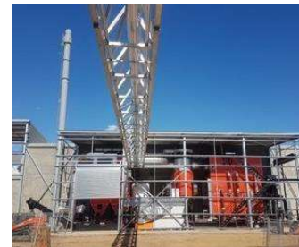
Biomass Steam & Hot Water Generation
