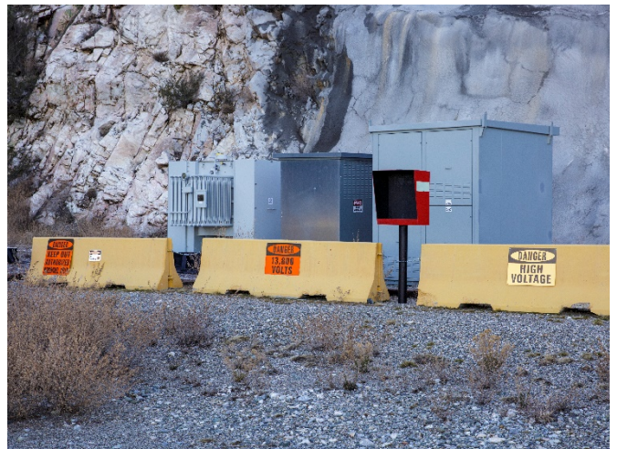
Photo 6 – Electrical Distribution Equipment on Surface
