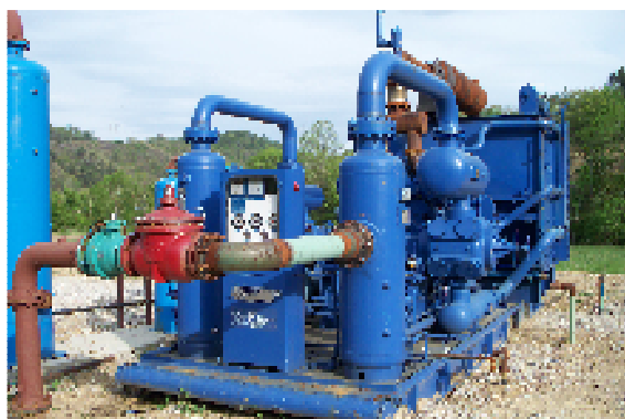
Gas Compression Plant owned by P&J Resources in Wayne County West Virginia.
