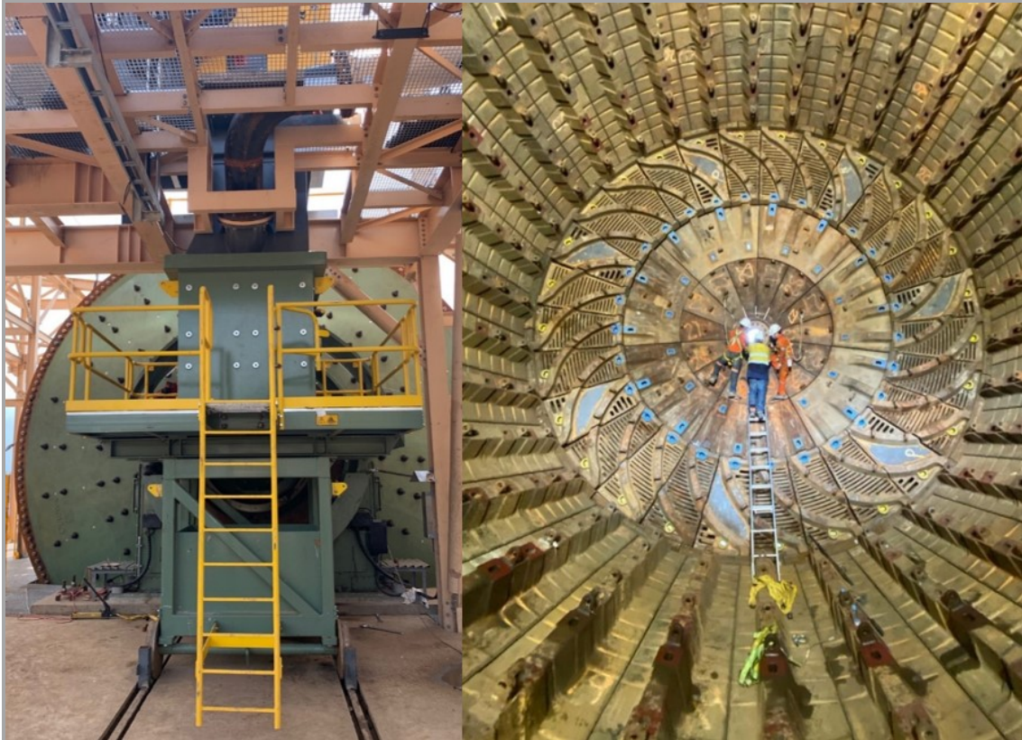
Figure 10 | SAG Mill – Commissioned and Operating
