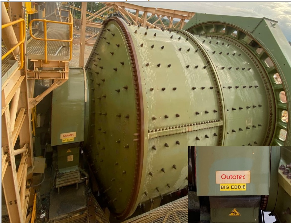
8 Megawatt Outotec SAG Mill "Big Eddie" named by Installation Engineer, P Nilsson in honour of his father
