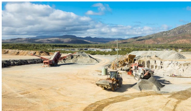
Figure 3 – Quarry Screening Plant
