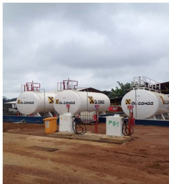
Figure 6: 50,000 Litre Fuel Storage Tanks at Mayoko
