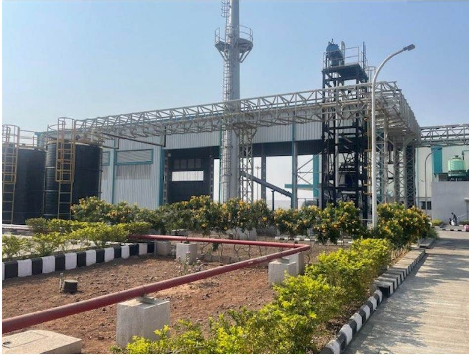
Figure 1 – Part of the expanded facility at PGT
