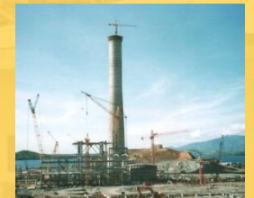
2 x 600 MW Sual Power Plant, the Philippines
