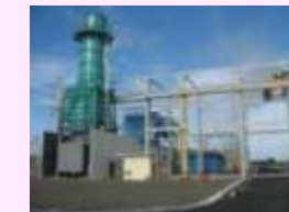
EWI - Power Station
