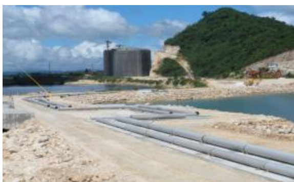
Stainless Steel Pipeline
