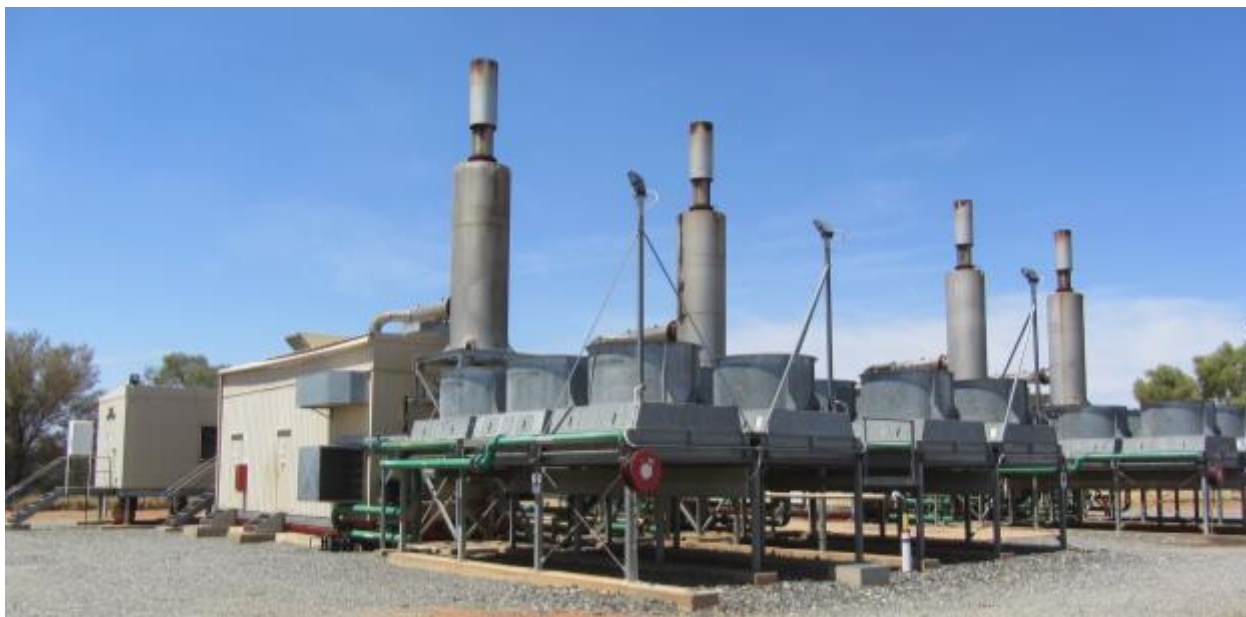
Alice Springs Power Plant, Australia
