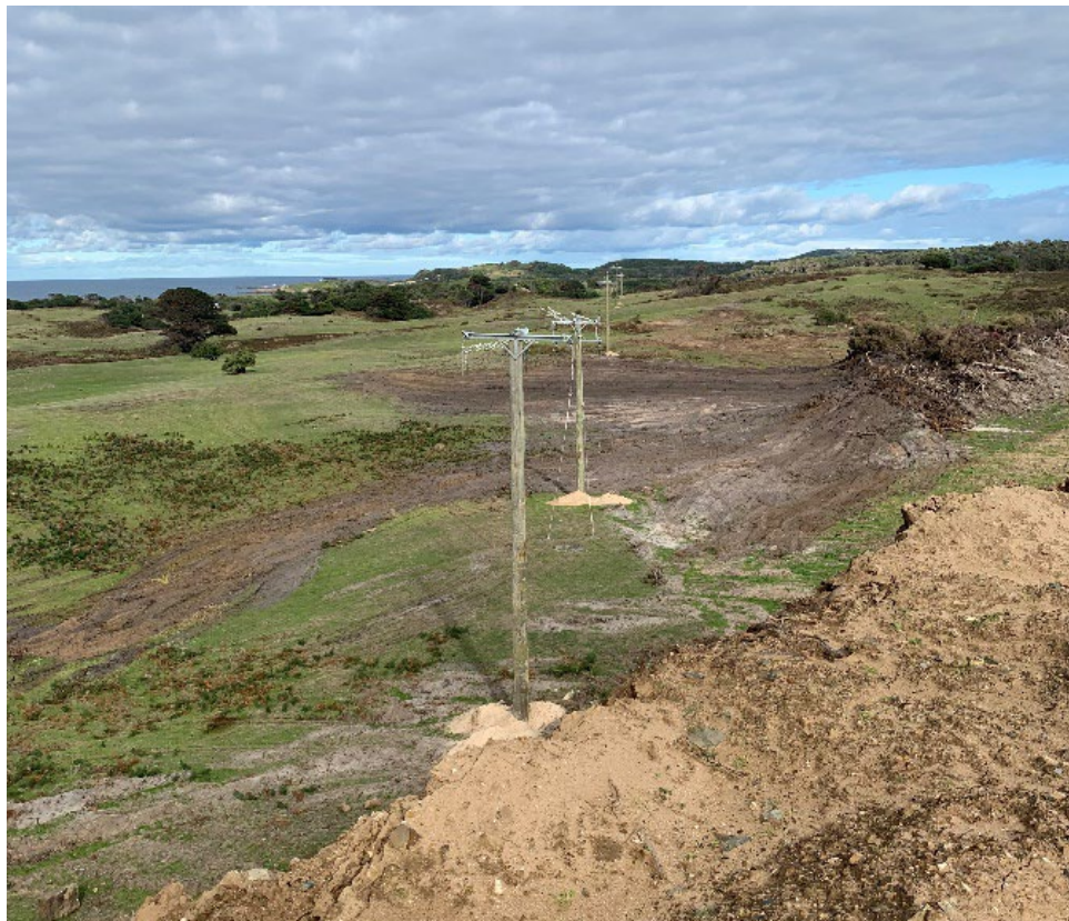
Figure 3. Overhead Power Connection from the King Island Grid
