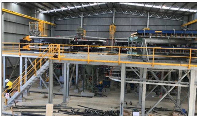
Figure 3 - View inside Process Building showing first floor gravity shaking table installation.
