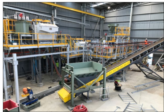
Figure 4 - View Inside Process Building looking east. With flotation area in the background and dryer feed conveyor in the foreground.
