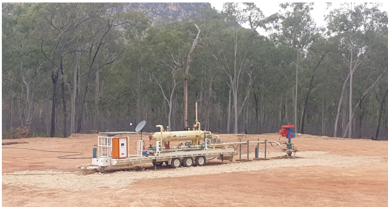
Gas production testing at Serocold-1, September 2020
