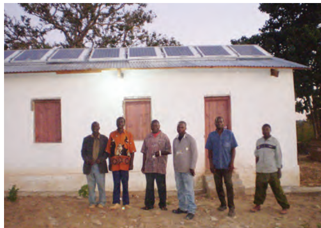
Installation of solar panels at Etandweni to run the lights and vaccine fridge
