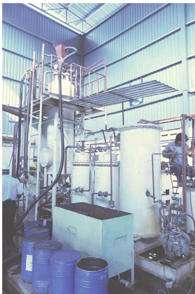
Photograph; Carbon stripping column.
