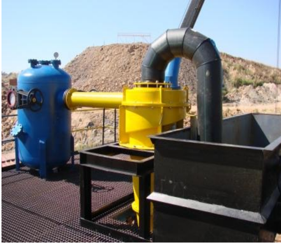
The TWT plant uses hydro cyclone technology during the first of two dewatering stages
