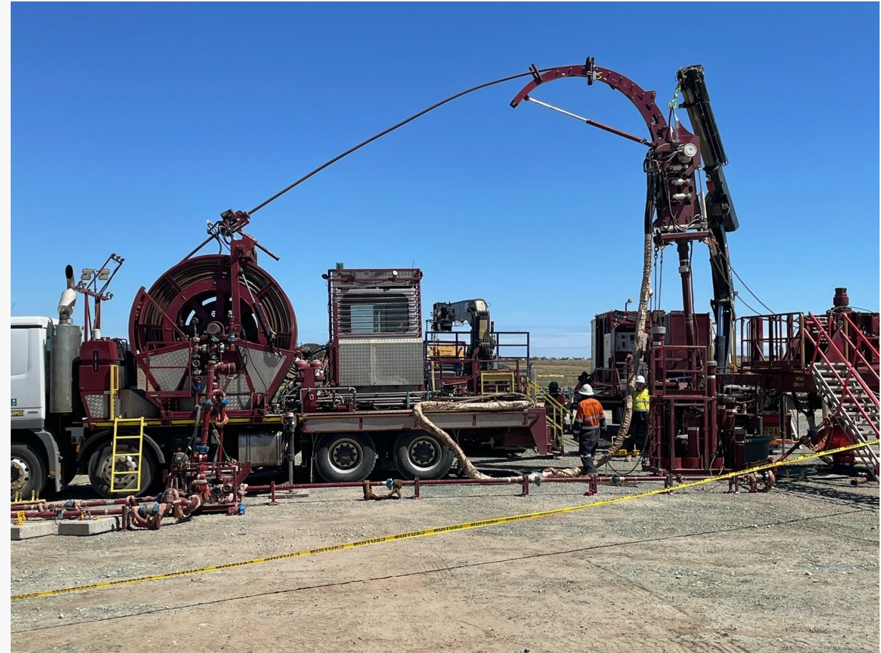
Well testing Equipment on Site at Ramsay 1
