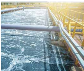
Wastewater treatment plant
