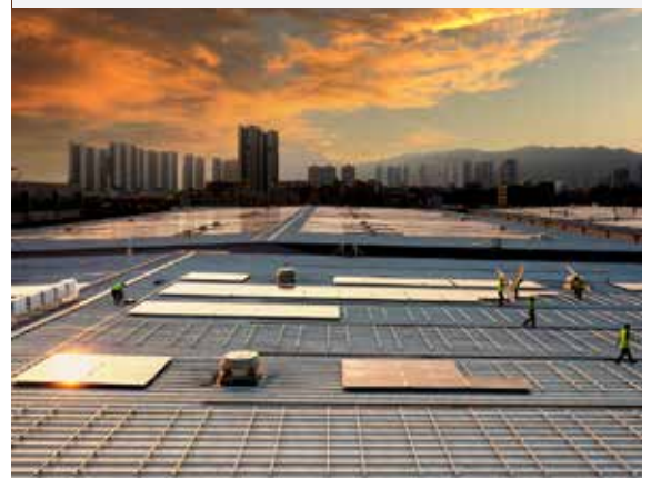
Goodman Huiyang Industrial Park, Huiyang, China.
