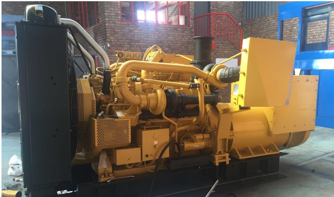
Figure 1: One of two 800kva Caterpillar generators recently purchased.
