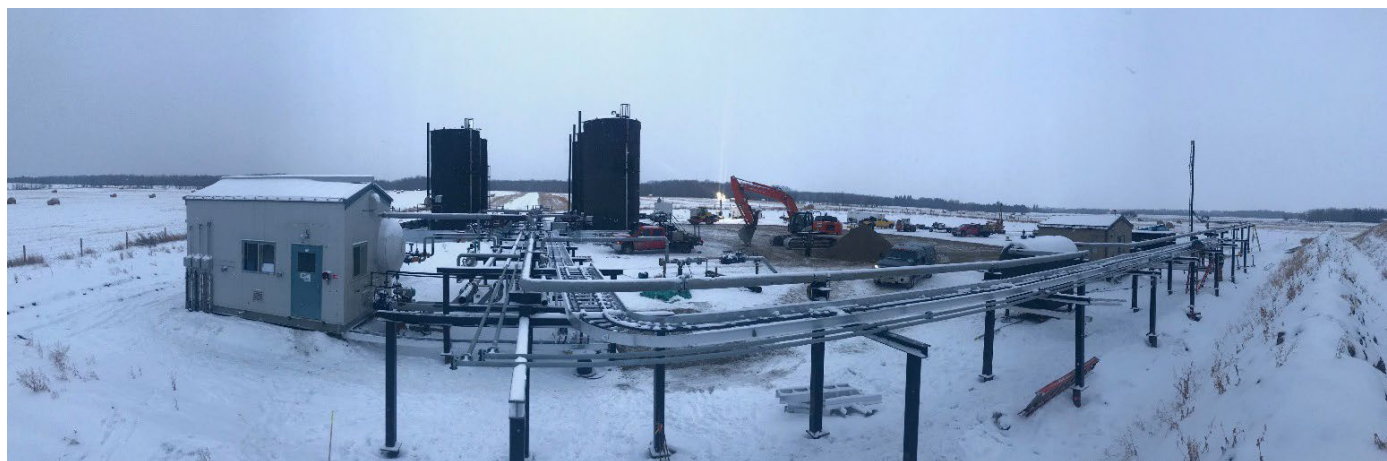
Figure 6 - Installed and commissioned upgraded Wizard Lake Facilities
