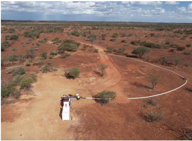
Figure 3. SipHon borefield in operation
