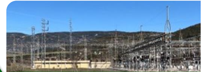
National Electricity Grid Substation in Sangüesa
