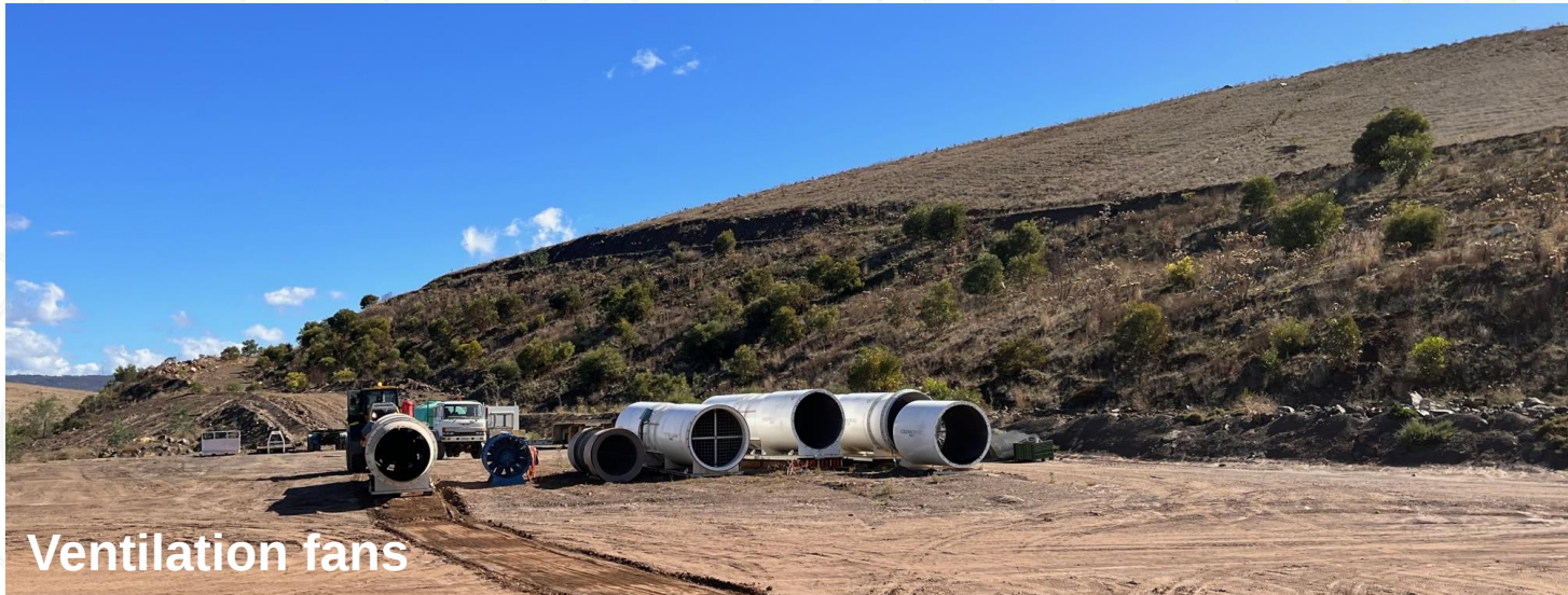
Primary ventilation substation
