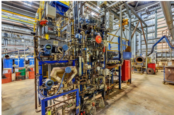
Figure 2: CSIRO Sintering & Pelletising Facility
