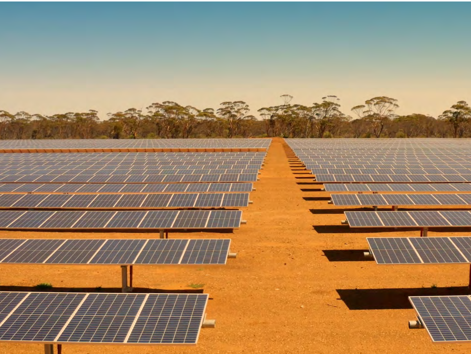
Nova Operation 5.5MW solar farm
