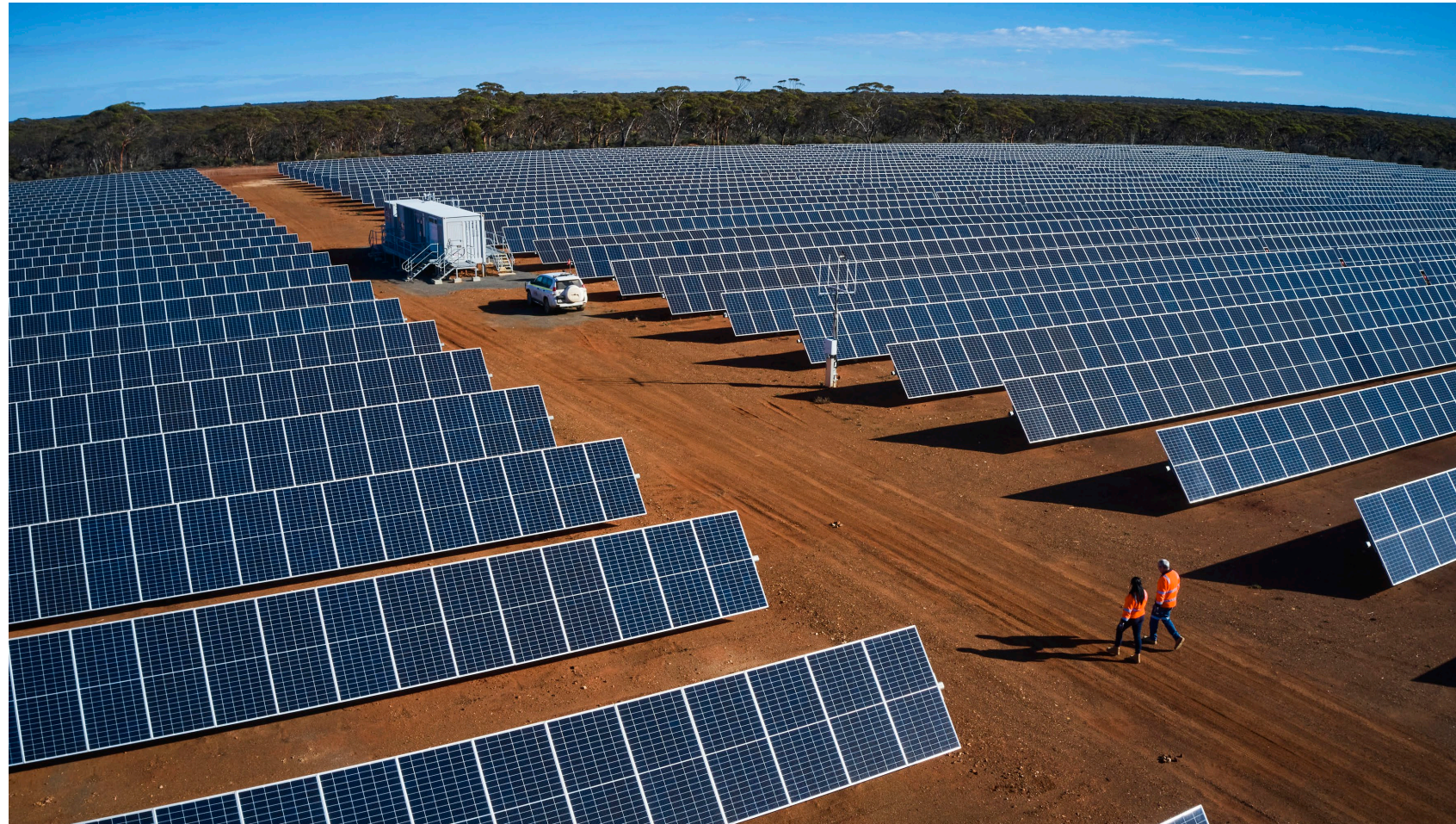
Nova 5.4MW Solar Farm
