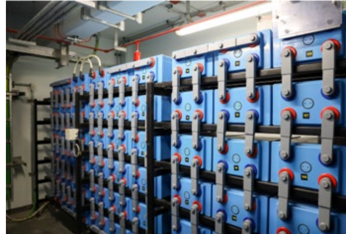
Renewable Energy Storage
