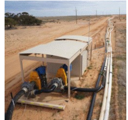
Slurry Booster Stations & pipelines
