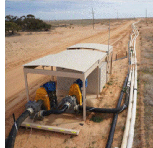
Slurry Booster Stations & pipelines
