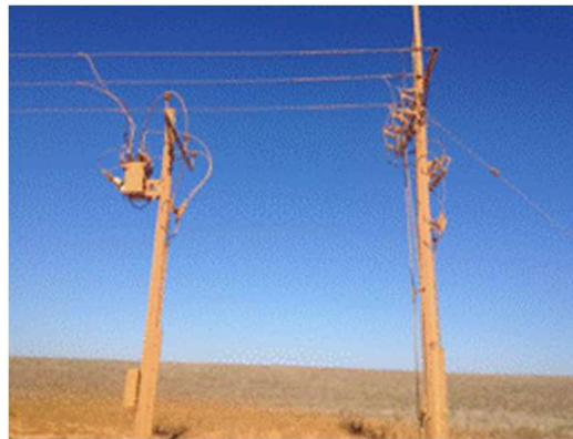
Power poles, wires & transformers
