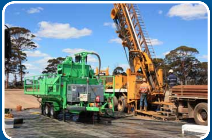
AMC Solids Control Unit
