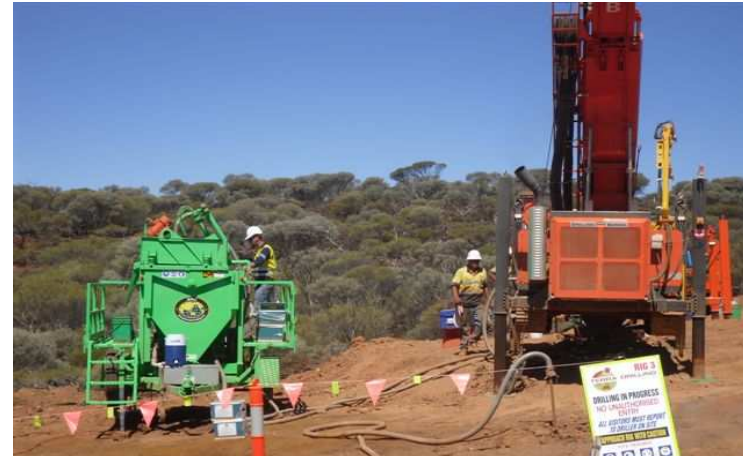
No sumps – fully enclosed system
