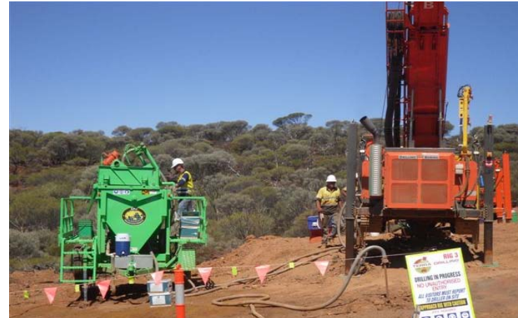
No sumps – fully enclosed system
