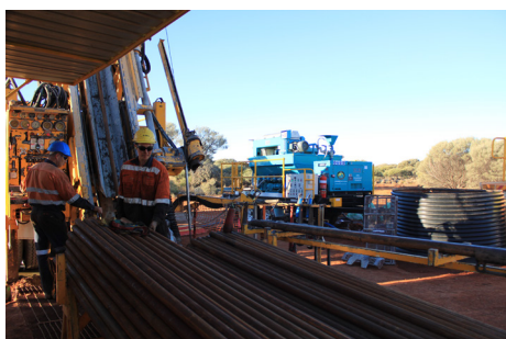
AMC SRU on site, Western Australia
