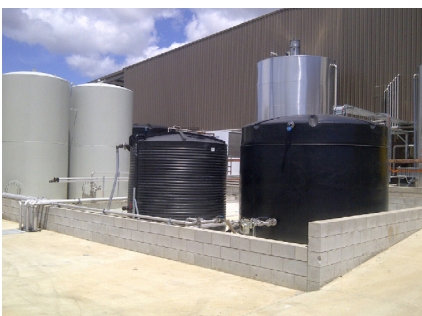
PHPA plant installed at Wildcat Chemicals
