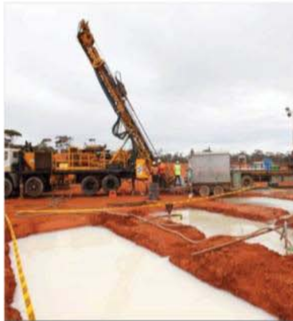
Traditional drilling fluid sumps
