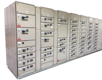
Medium Voltage Distribution
