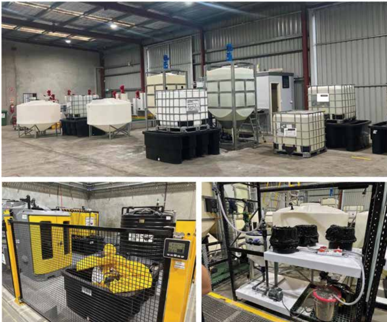
Figure 1.11. The HiPurA pilot plant: note the filtration units still in wrappers.
