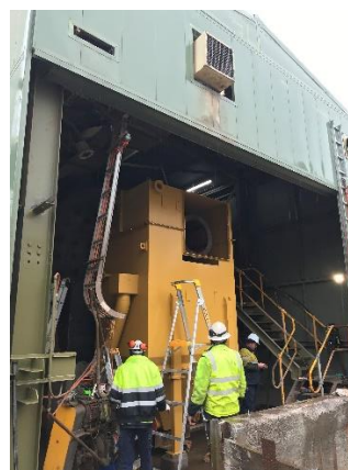
Figure 2. New SAG discharge hopper
