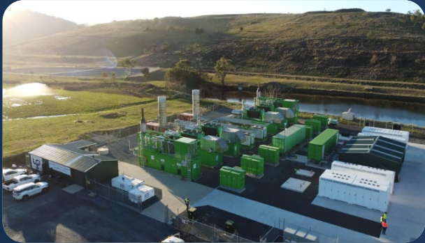
Batteries at Canberra
