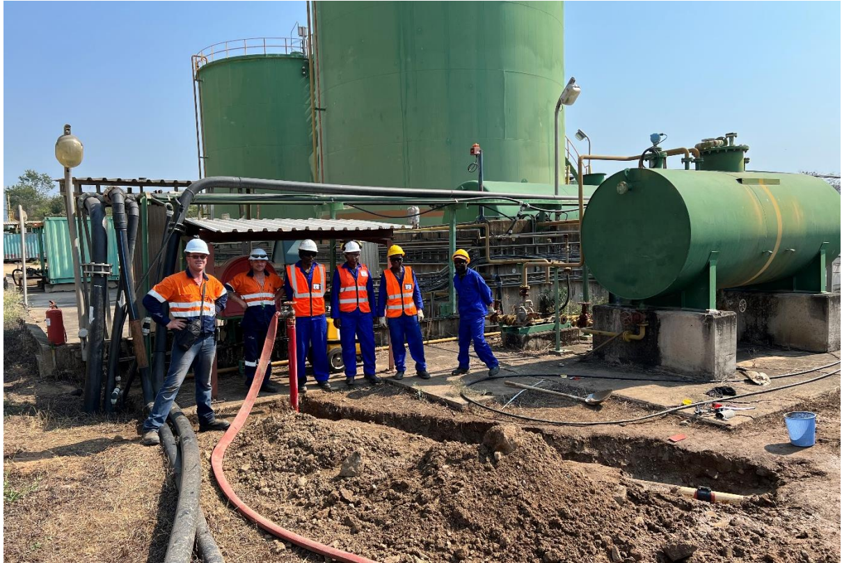
Figure 4: Fire water system upgrade
