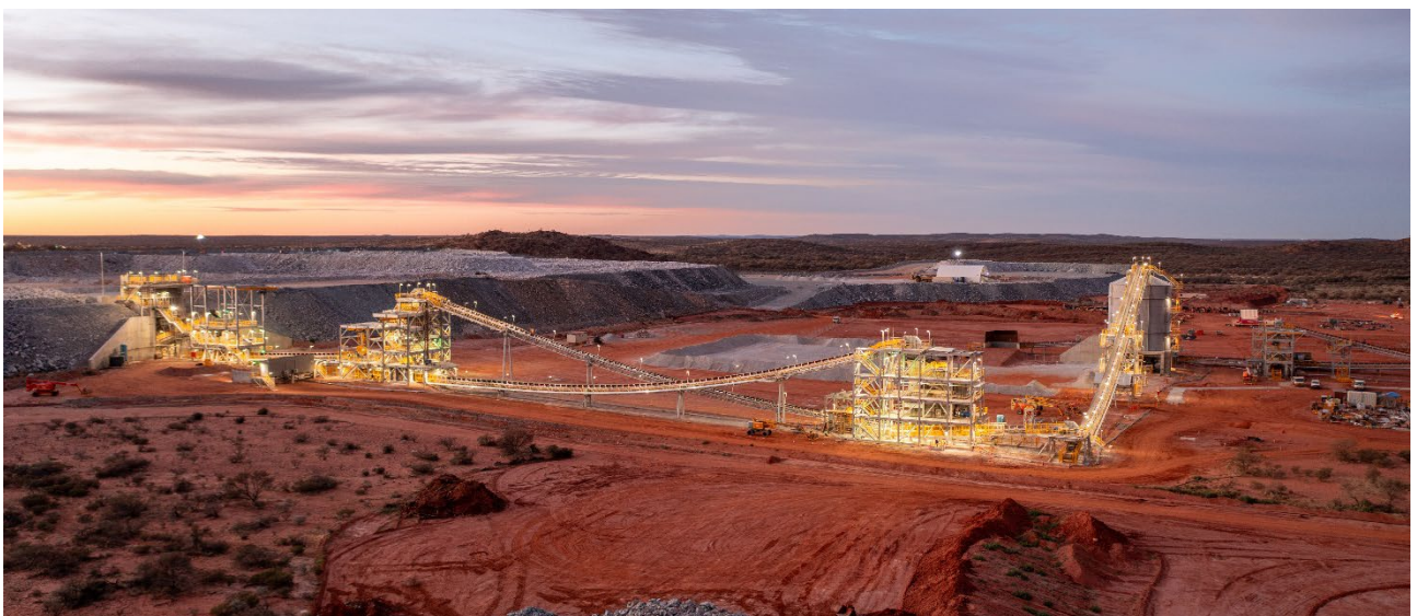
Figure 14: Side view of Crushing Plant
