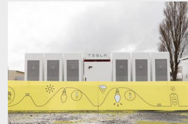
Hugo Johnson Drive - Battery 1MW / 2MWh (2018)
