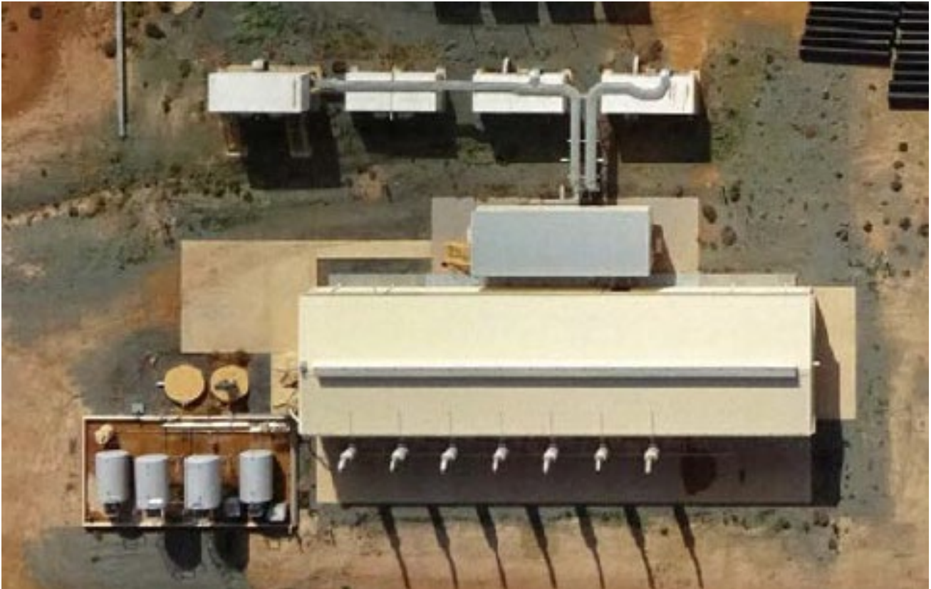
Figure 52 – Andy Well power station (generation units and switches need to be reinstated).
