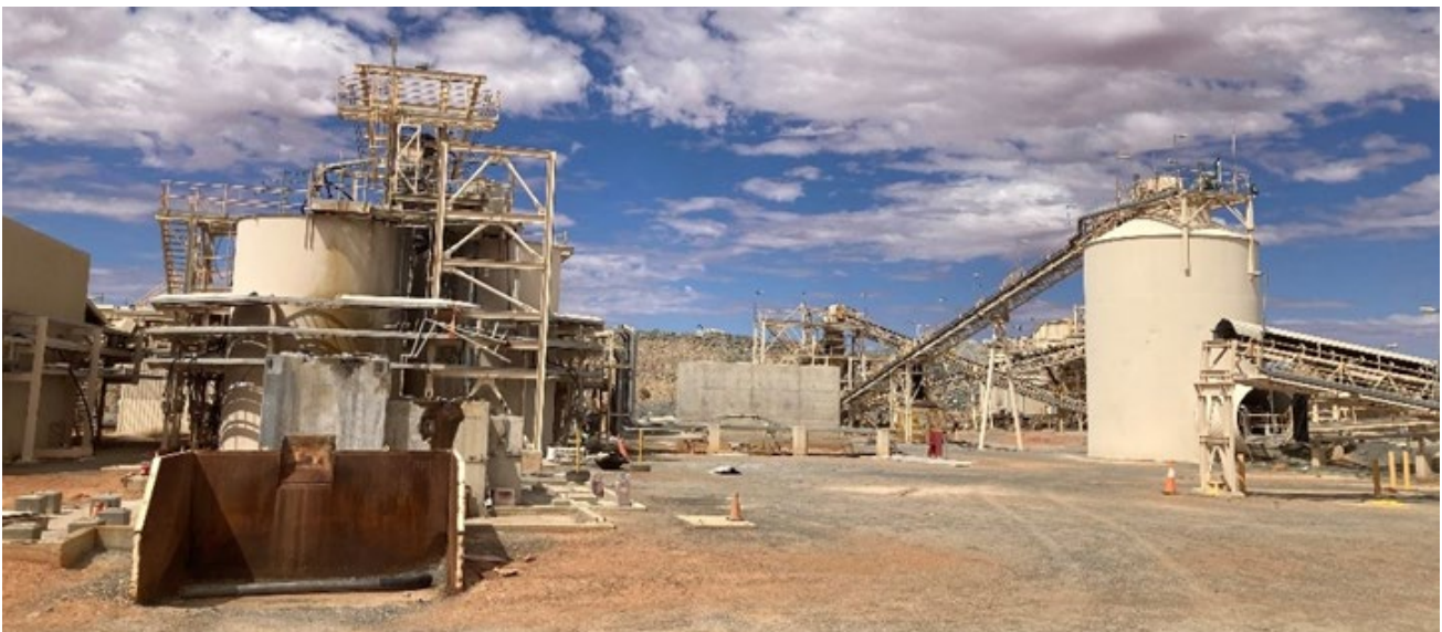
Figure 40 – View of grinding area, ball mill plinths and scats bunker (ball mill removed).
