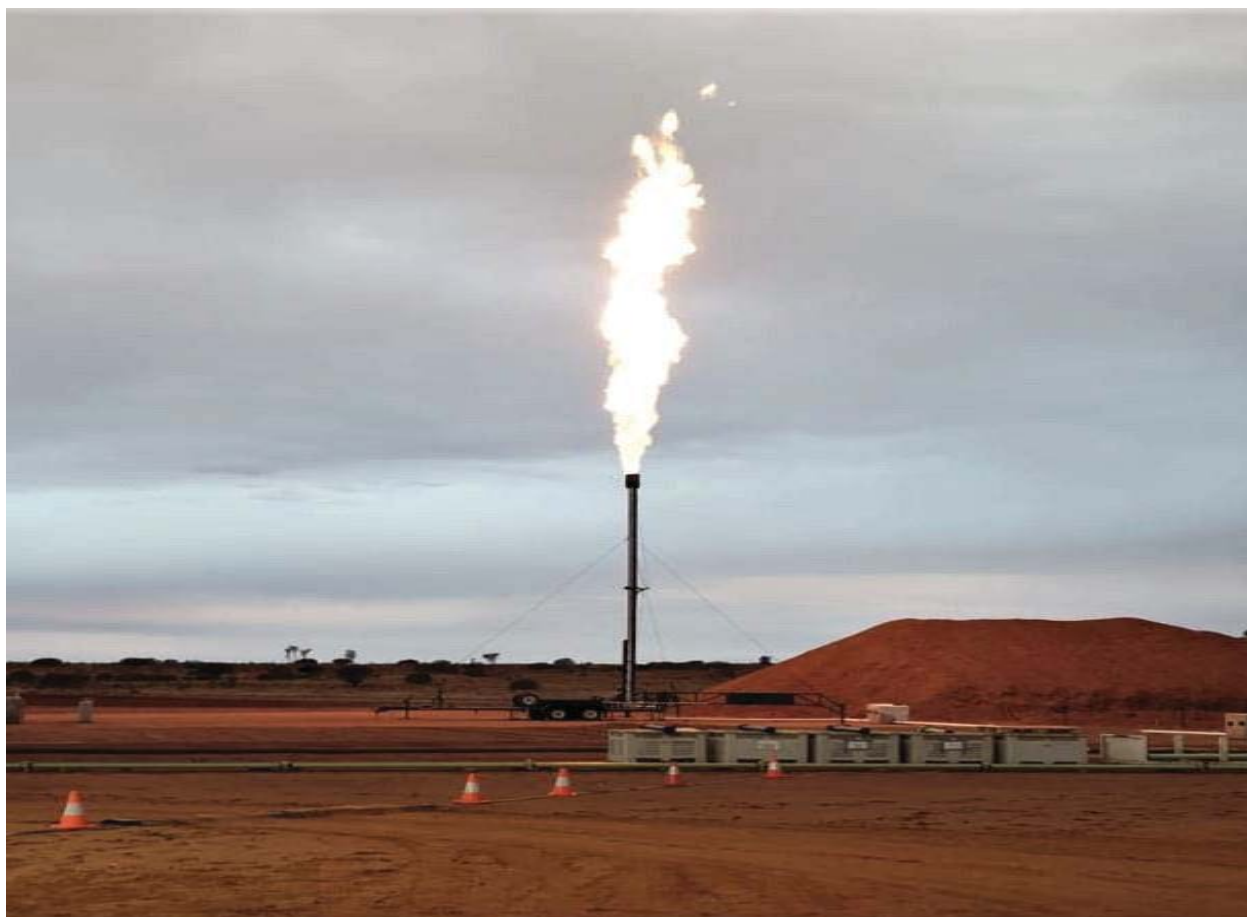
Figure 2: Gas Flare at Vali-1 ST1(5 August 2020)
