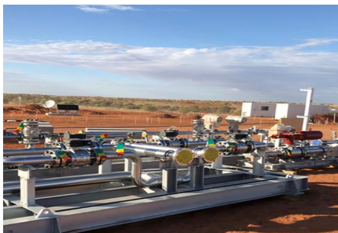
Skids at separation and metering lease ready for installation
