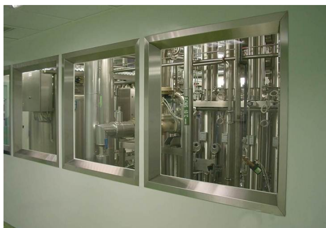
Water for Injection Plant
