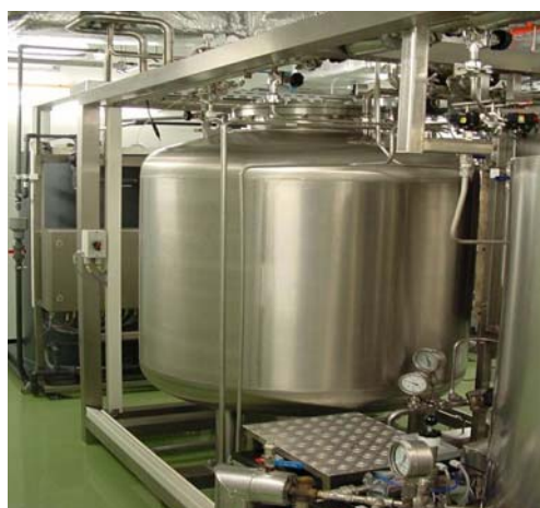
Reverse Osmosis Water Tanks
