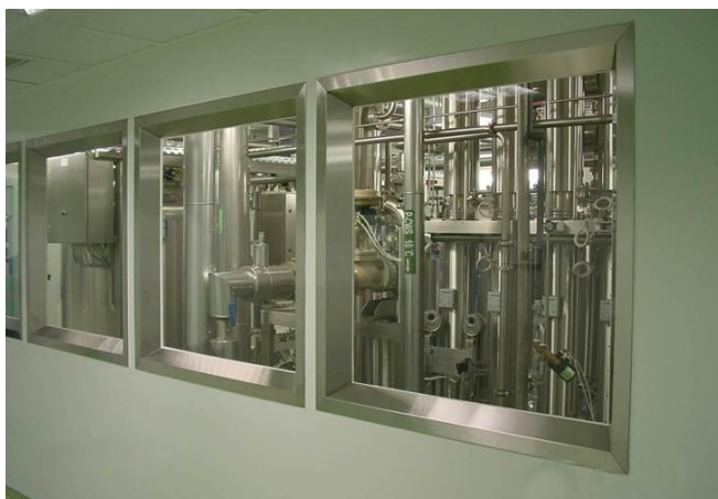
Water for Injection Plant
