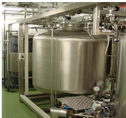
Reverse Osmosis Water Tanks
