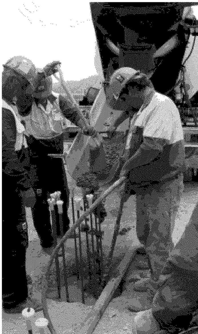
First concrete is poured for the Foundry at the Stanwell Magnesium Plant
