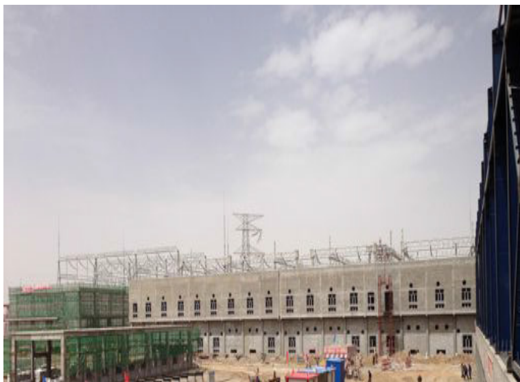
Transformer building (adjacent to cell house)
